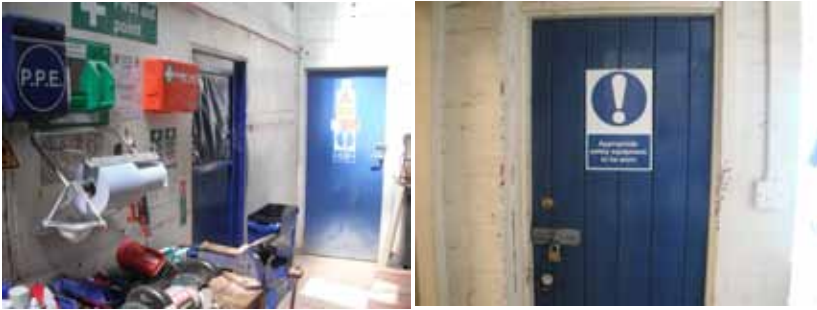
Inside the old Boiler House and the door leading to the shower
